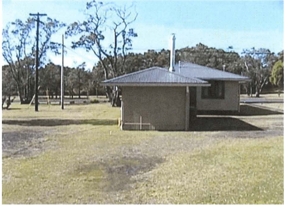
Plate 20. Construction area on the north side of Bldg. #64 (Bldg. 63 in the background).
